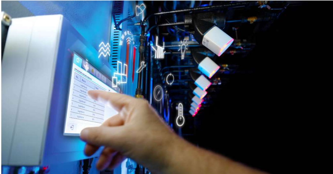
The Hycleen Automation System digitally retrofitted thanks to the akenza platform. Image credit: GF Piping Systems
